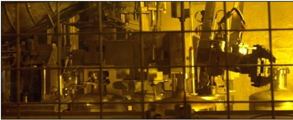
View through protective shielding of DWPF Melter Cell showing a canister being filled.
