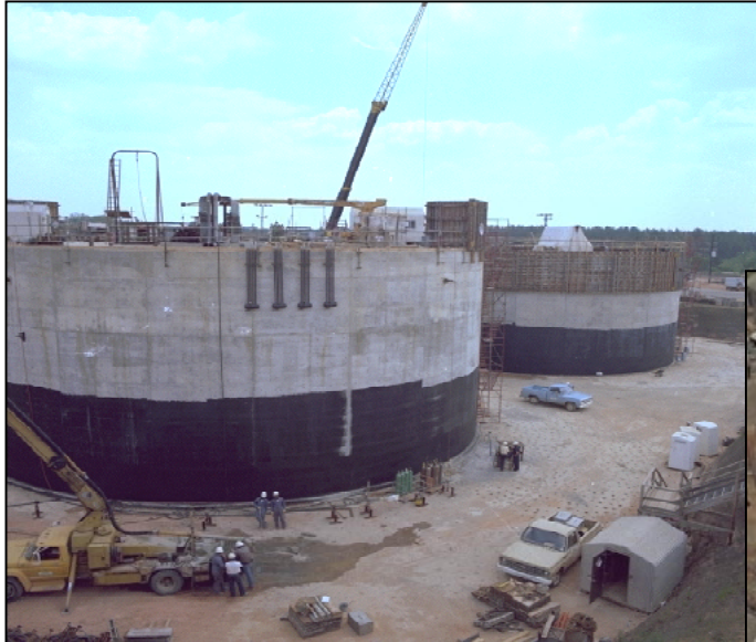
Tanks under construction. Note tank size relative to construction workers. Later, dirt is backfilled around the tanks to provide shielding.
