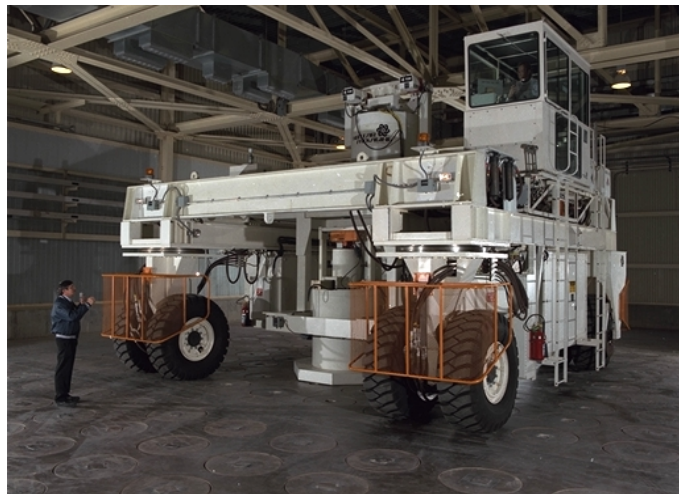
The Shielded Canister Transporter (SCT) moves highly radioactive canisters from DWPF to the GWSB. The SCT removes a round shield plug from the floor, lowers the canister into a vertical storage position, and replaces the shield plug.
