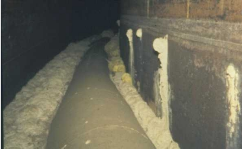
Tank Annulus showing High Level Waste that has leaked from the Primary Tank in the past and has solidified
