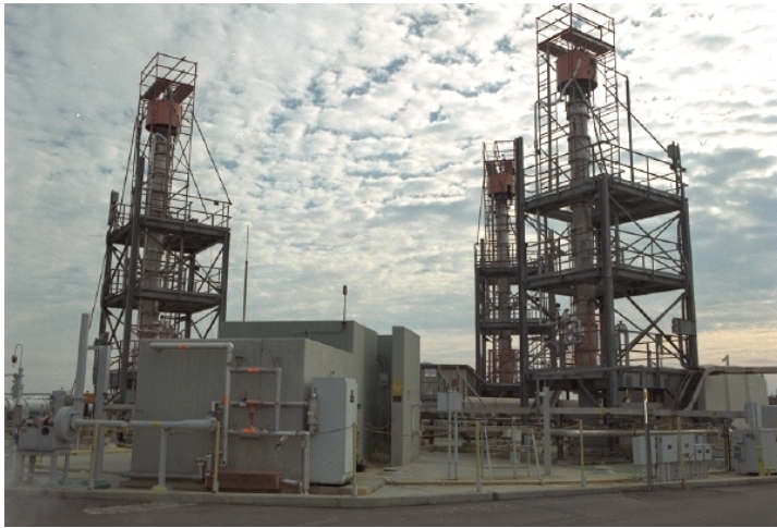
Typical Waste Removal equipment includes three to four 45-foot long slurry pumps and one transfer pump or jet. Note the substantial structural steel required to support the loads in the picture above. At right is the typical installation of a transfer pump (Tank 8) requiring difficult, high-risk equipment entries into High Level Waste Tanks.
