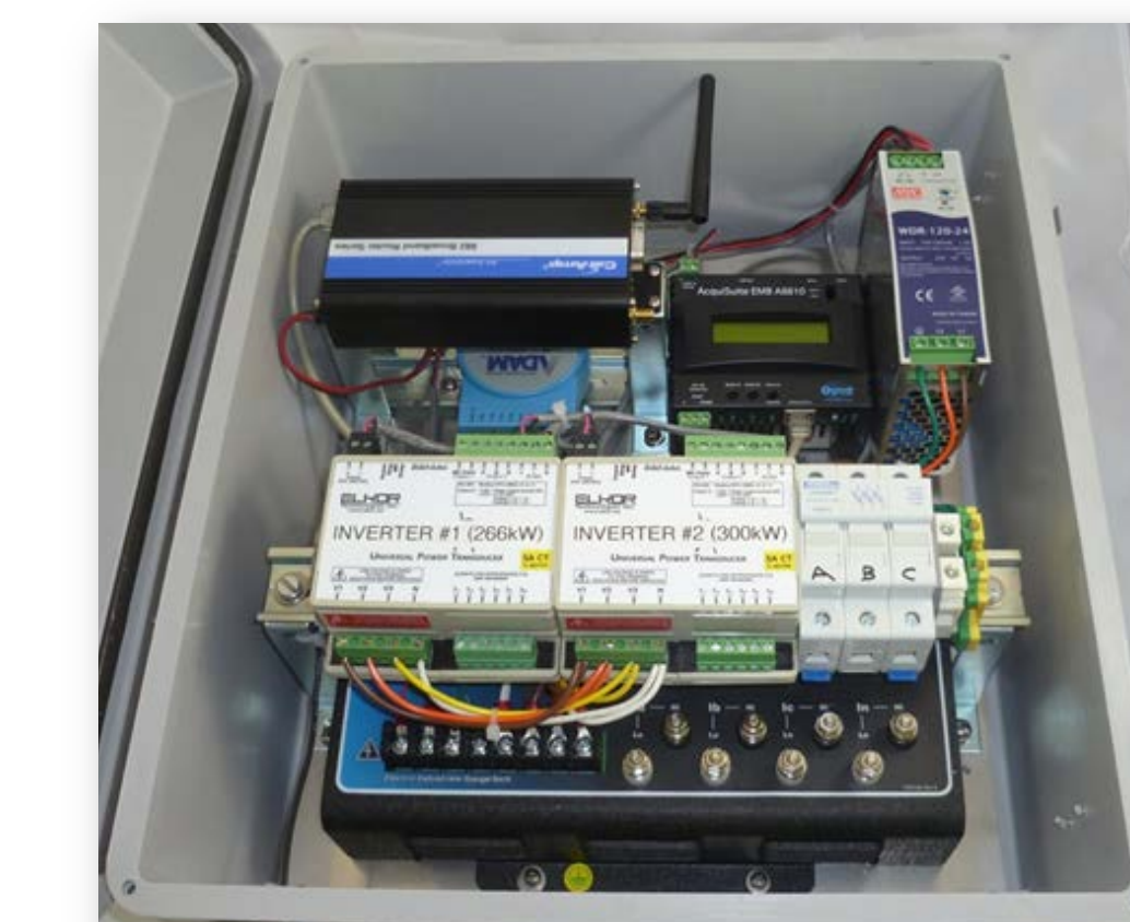
Solar PQ Monitoring System
