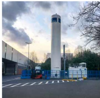
Fuel cell forklifts fueling station
