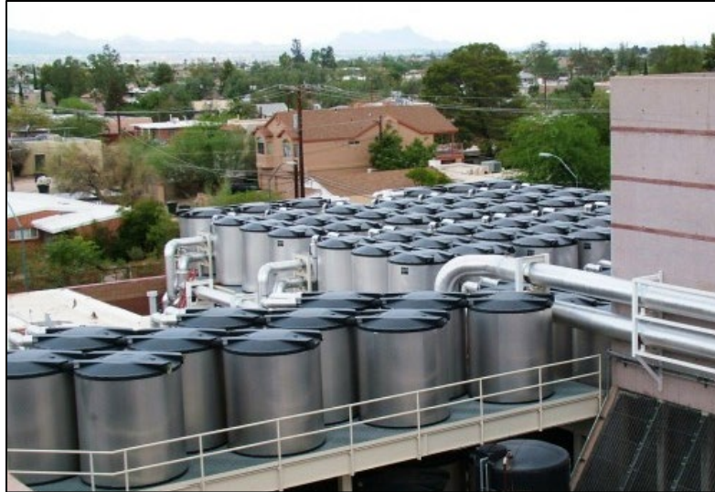
Figure 57. Thermal energy storage installation
