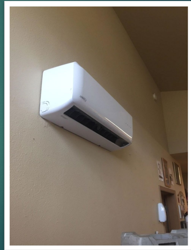
New Heat Pump – inside view
