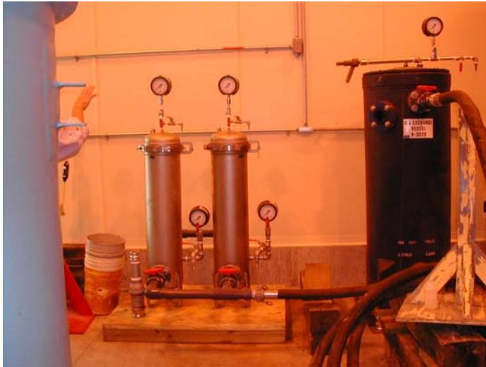
Photo 21. Ion Exchange system for leachate treatment.
