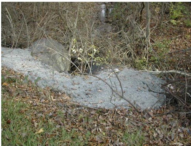
Photo 11. Inlet side of Highway D Culverts. Concrete had been placed on outside and in the middle of culverts.
