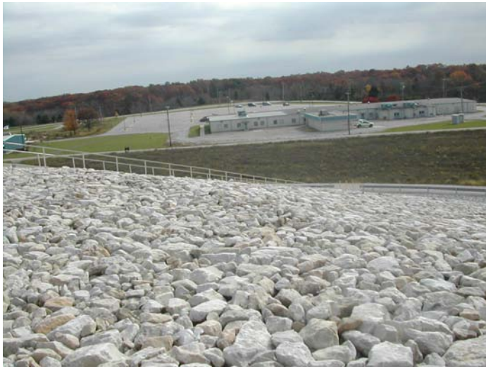
Photo 18. View from top looking SW towards admin bldg. Slight bulge.
