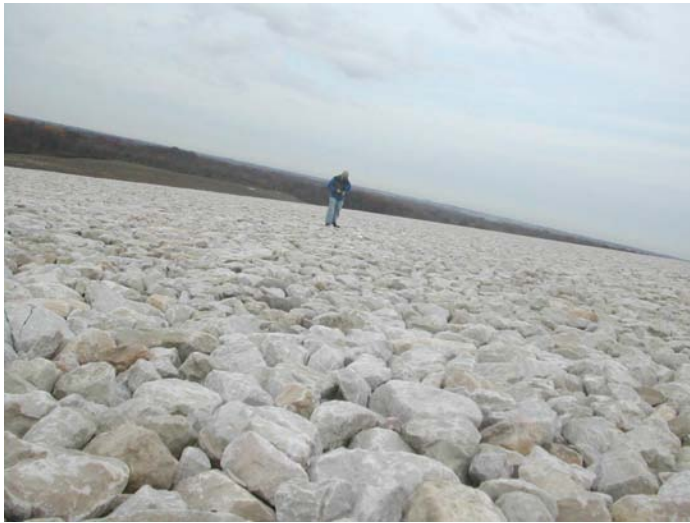
Photo 19. Slight depression area shown on aerial survey on southwest side looking northwest.
