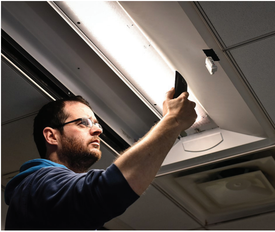
An installer uses a cell phone to configure the system. All but two of the systems ultimately required factory assistance during installation or following setup.
