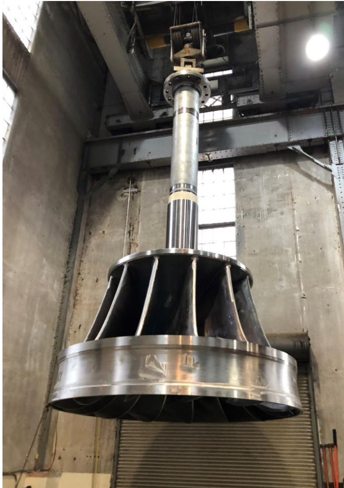
New GE Aerating Turbine installed at Cube Hydro's High Rock Hydropower Project
