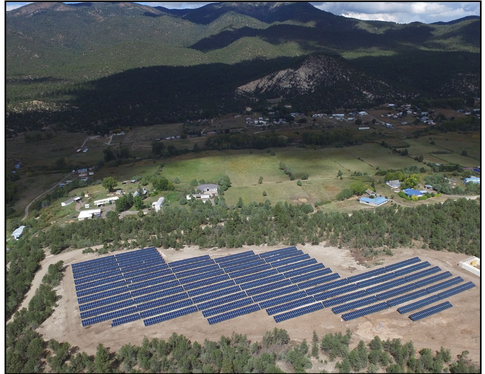
Picuris Pueblo (NM) completion of the 1 MW solar photovoltaic system (October 2017)
