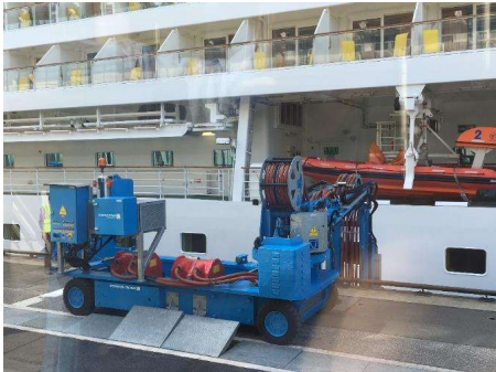
Stationary onshore power supply for both cruise vessels (in operation) and container vessels (planned)
