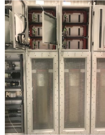
Variable Frequency Drive System FAT setup
