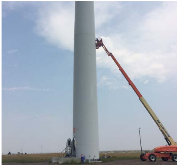
Installation on GE 1.5 MW wind turbine at the NWTC (Photo by Bethany Straw)
