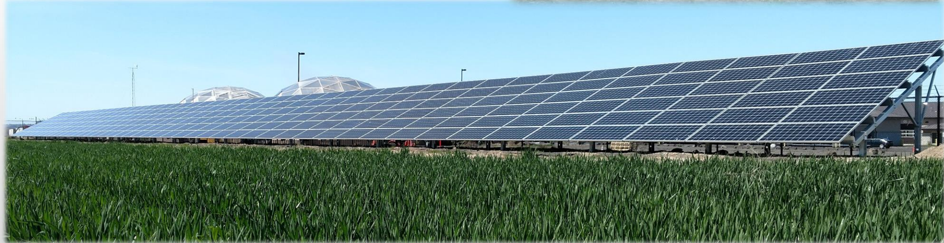
(Top) CTUIR and Elemental Energy staff preparing to install the final solar module (Bottom) The completed Ántukš-Tiñqapapt (“sun trap”) Solar PV Array
