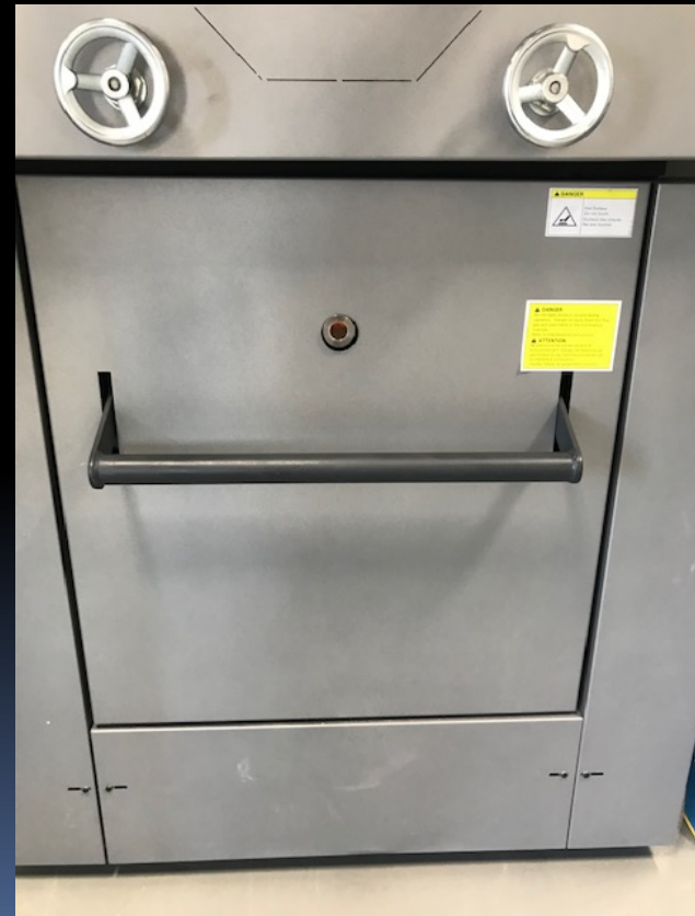
The BOILER gets commissioned
