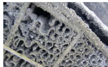
Mineral buildup on cooling tower fill
