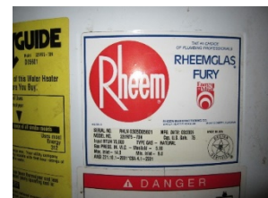
Hot water tank nameplates with make and model
