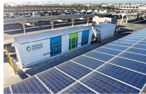
Early version of EnergyPod installed at MCAS Miramar.
