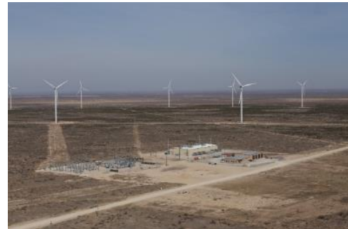
Wind storage demonstration system with wind turbines in the background
