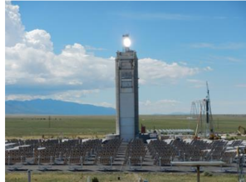
Falling Particle Receiver installed at the National Solar Thermal Test Facility at Sandia National Lab to evaluate proppant (sand-like ceramic particles) as the heat storage medium.
