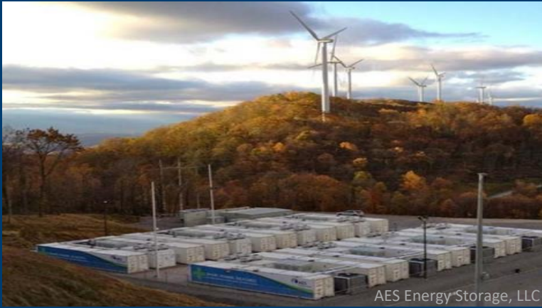
AES Energy Storage, LLC
