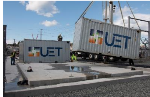
Snohomish PUD's flow battery system housed in shipping containers. Batteries manufactured by UniEnergy Technologies.
