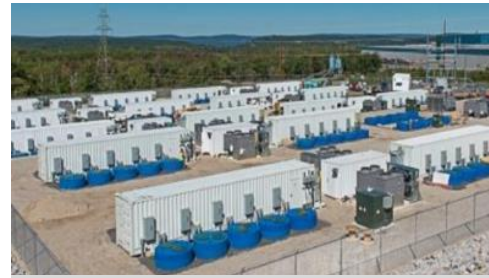
20-MW flywheel facility in Hazle, Pennsylvania
