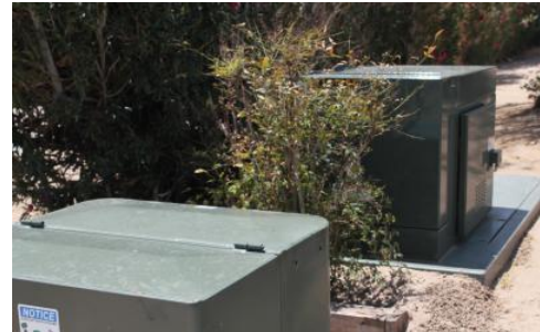
Distributed residential storage for the Borrego Spring MicroGrid—the first of its kind to power an entire community with renewable energy.
