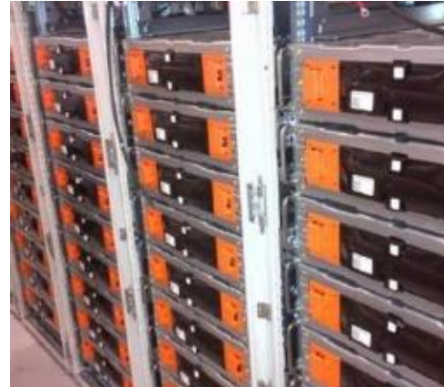
Energy Storage equipment for wind storage project
