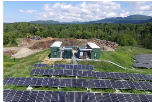
Stafford Hill Solar and Battery system in Vermont
