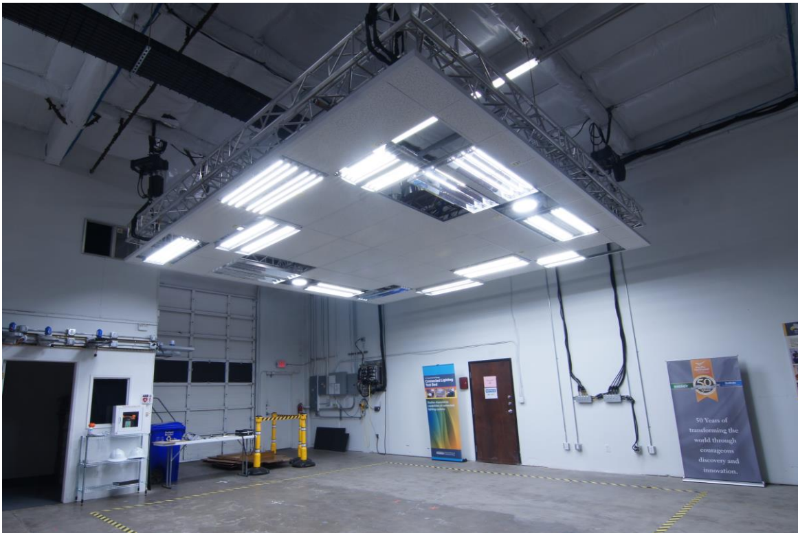
Figure ES.1. Mockup space with all seven pairs of Top Efficacy Performer luminaires installed and energized.
