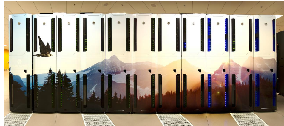
NREL's Peregrine supercomputer: Capable of 2.2 PetaFLOPS. Photo by Dennis Schroeder, NREL 27774
