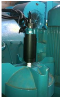
Compact filter testing
