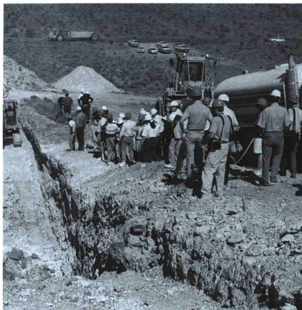
Preliminary digging begins on July 8, 1991, for Yucca Mountain site evaluation following the State of Nevada's issuance of an air quality permit.
