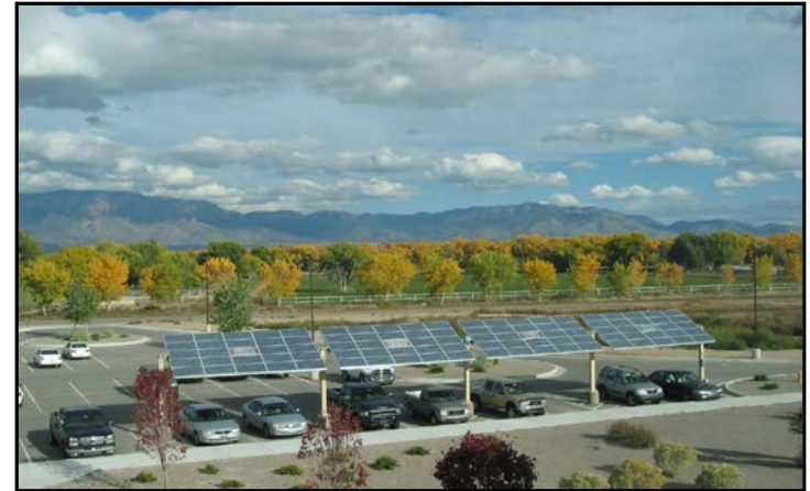
PV System (6 kW) at SIPI's (NM) Science and Technology Building
