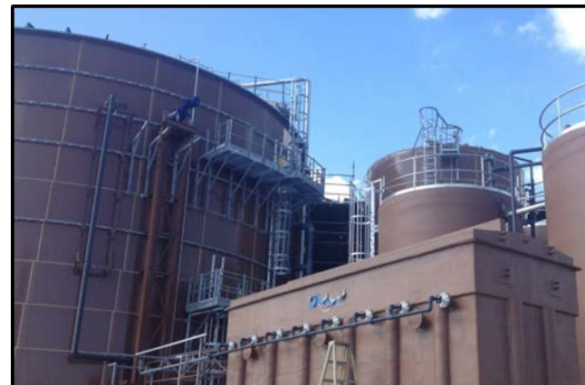
Forest County Potawatomi Community(WI) 2-megawatt anaerobic digestion and biogas generation facility (May 2013)
