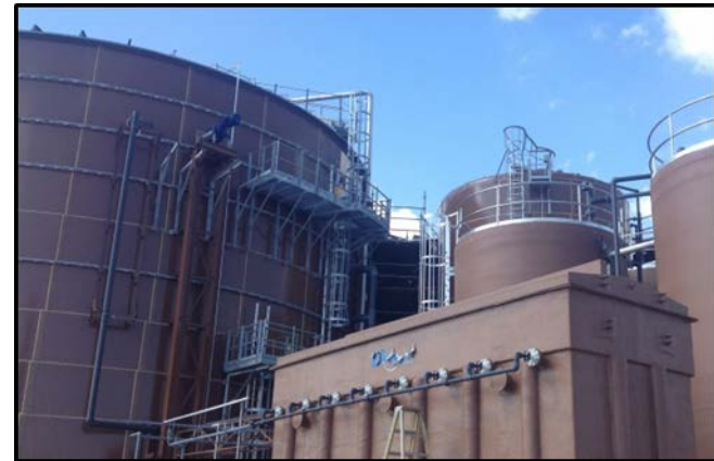
Forest County Potawatomi Community (WI) 2-megawatt anaerobic digestion and biogas generation facility (May 2013)
