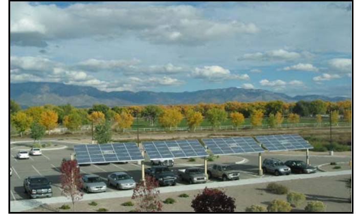
A 6kW PV System at SIPI's Science and Technology Building (NM)
