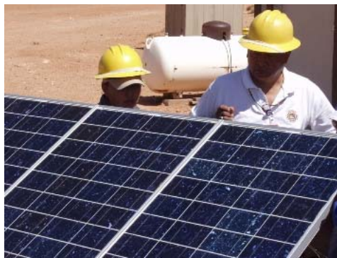
Figure 4 NTUA's Larry Ahasteen and electrician inspect PV system 18
