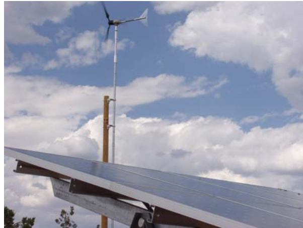
Figure 5 PV-Wind hybrid system on Navajo Reservation 22
