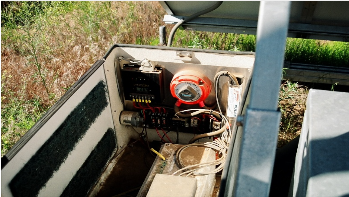
Figure 6. Inside the NTUA PV System Box
