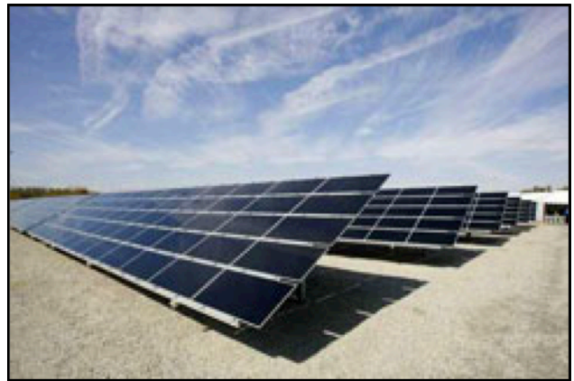
Augustine Band's 1.1 MW solar PV array in Southern California Photo source: www.epa.gov
