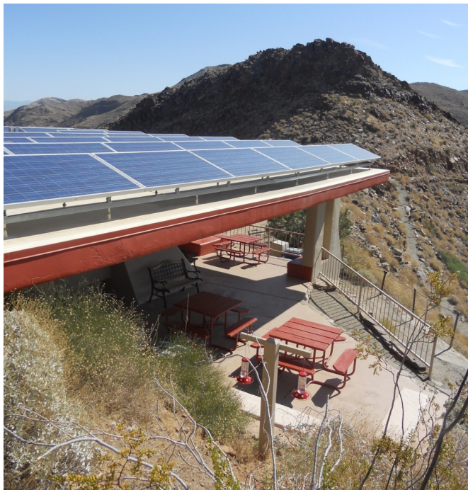
Photo showing Trading Post after PV installation, taken from Southwestern view. Source: Sandra Begay-Campbell
