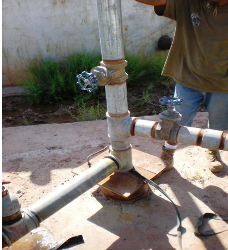
Figure 7: Main line at well site diverging to the fields and storage units.
