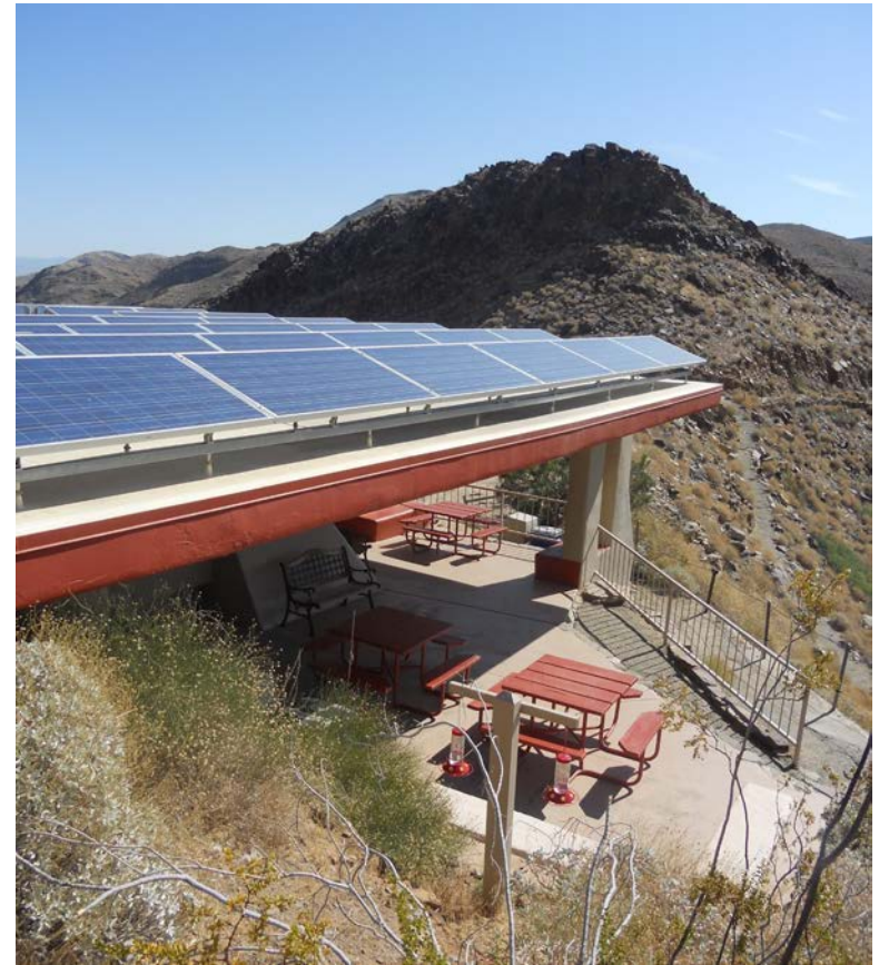
Picture showing Trading Post after PV installation, taken from Southwestern view. Source: Sandra Begay-Campbell
