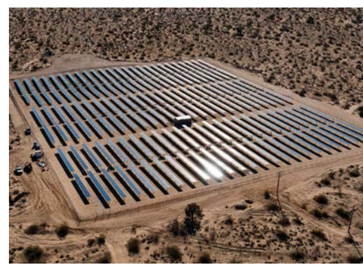
1-X Tracking Ground Mount PV
