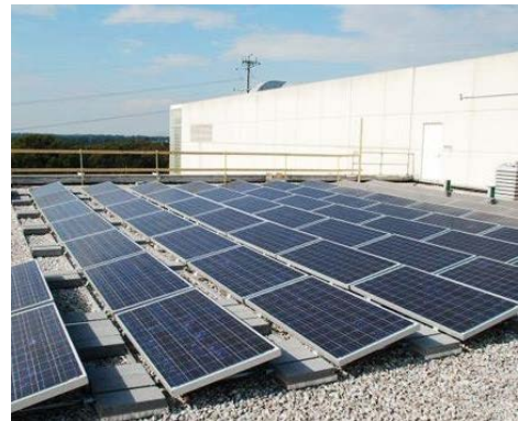
Fixed Tilt Roof mounted PV
