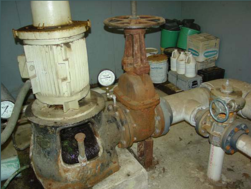
1 x 15 HP Deep Well Pump in Water Resources Office
