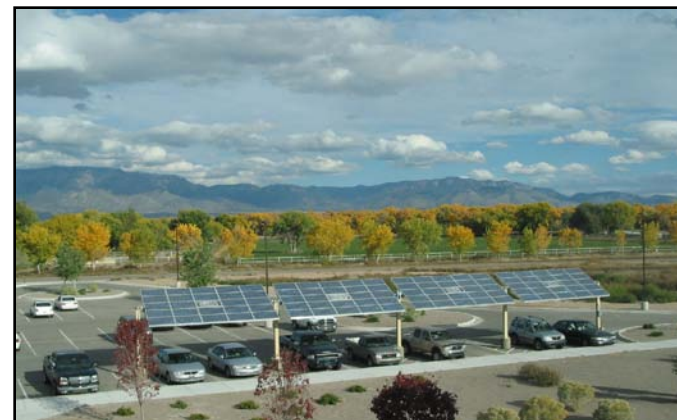
A 6kW PV System at SIPI's Science and Technology Building
