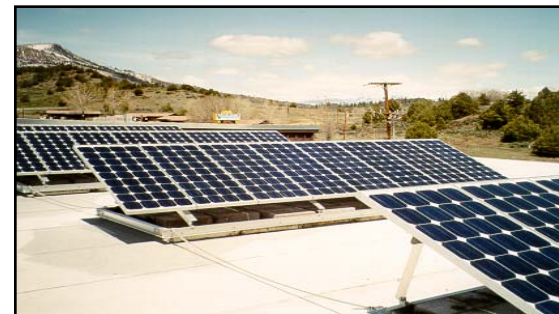
Jicarilla Apache Reservation PV array on Dulce High School
