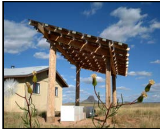
Solar arrays on Navajo home (AZ)
