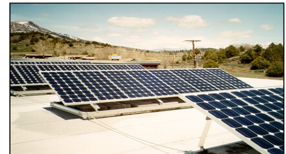
Jicarilla Apache Reservation PV array on Dulce High School (NM)
