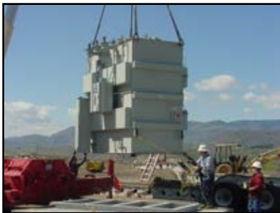
Colville Indian Power and Veneer Energy Substation (WA)
