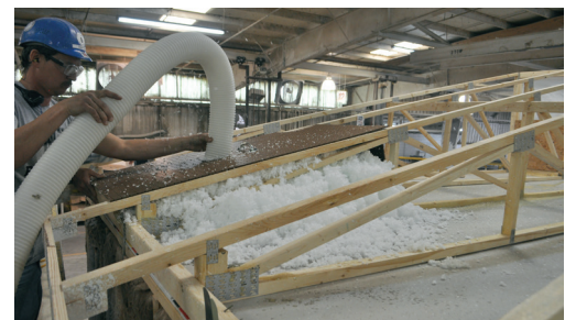
Installers start at one end of the house and work their way down, filling one bay at a time in about 23 seconds per bay.
