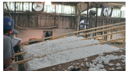
After all of the eaves are dense packed, the remainder of the attic is filled with loose fill to the desired height.
