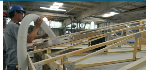
An employee at Clayton’s Southern Energy Homes plant uses a perforated hardboard “mold” to dense pack blown fiberglass insulation into the eaves of a manufactured home. The light-weight mold is 4 feet long and just wide enough to span the rafter bay with a hole in the middle for the insulation tube. A flange at the far end holds the insulation in place as it is blown in.
