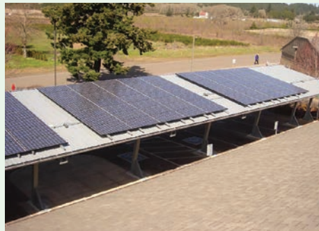
PV panels installed on Grand Ronde Tribal Housing Authority carport. Photo from GRTHA, NREL 31797
