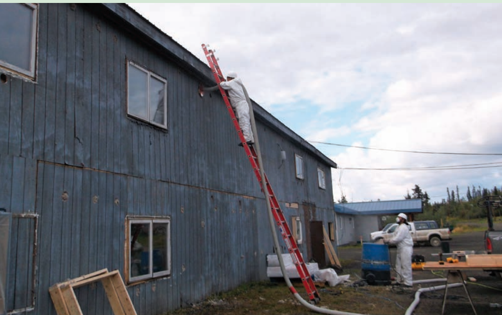
With DOE support, workers weatherize the exterior of the Lakeview Lodge in Minto, Alaska. Photo from Russell Snyder, Interior Regional Housing Authority, NREL 31796
