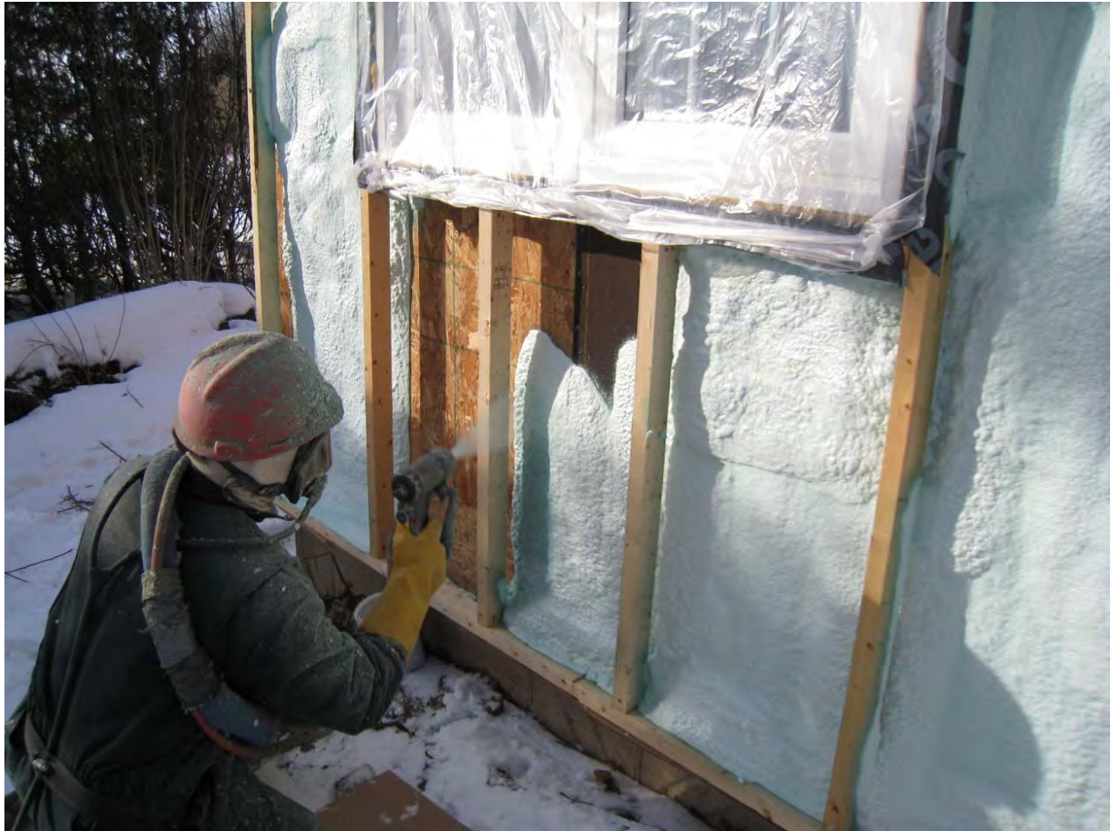
Figure 15 : Installation of high density spray foam in an Offset Framed Wall in a cold climate
