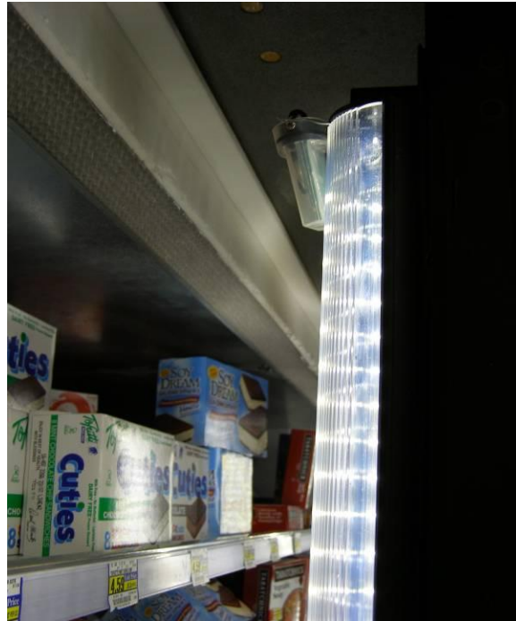
Figure 6. Hobo Light Level Logger installed at top of new LED light strip.
