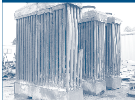
Figure 1. Example of a poorly maintained heat exchanger from an aluminum melting furnace
