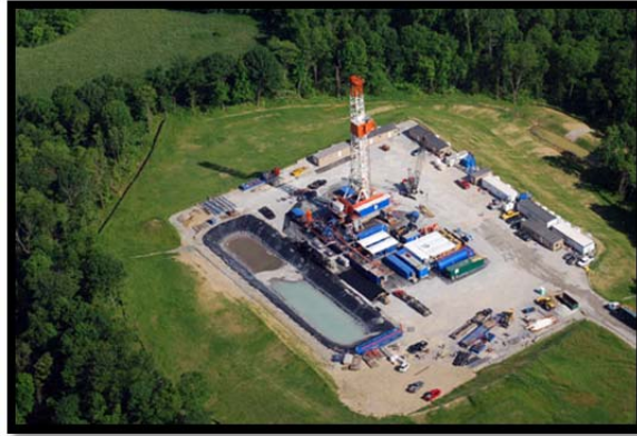
Figure 18: A Typical Well Pad in Pennsylvania (Photo courtesy of Robert M. Donnan, http://www.marcellus-shale.us/ )
