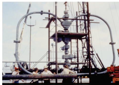
Figure 28b. To accommodate the high brine flow rate, a block “Y” was installed on the production wellhead.
