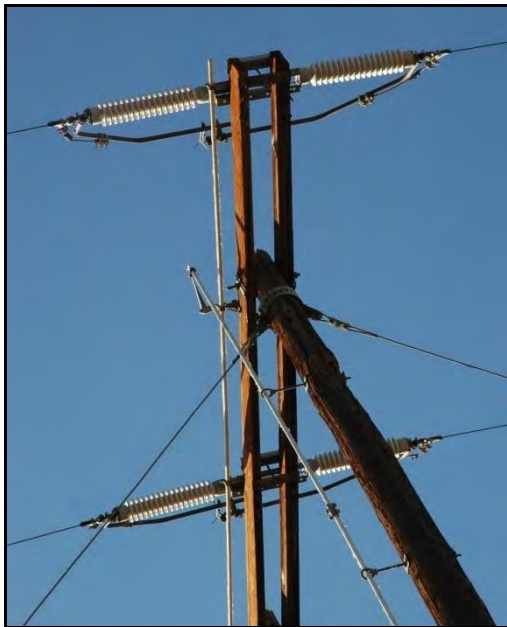
Photograph 1-1 Example of a Switch
