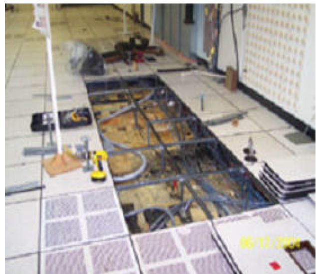
Exposed CO 2 Fire Suppression System
