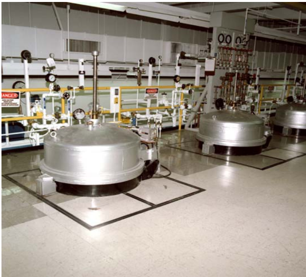
Y-12 Process Equipment
