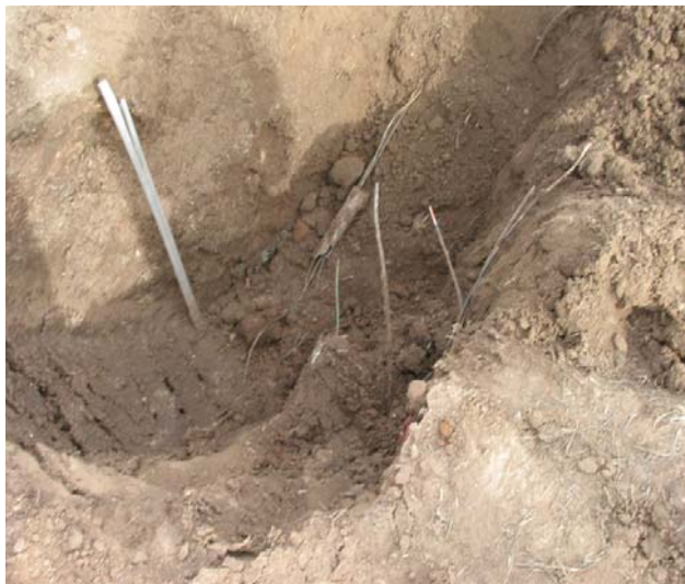
Buried Electrical Line Cut
