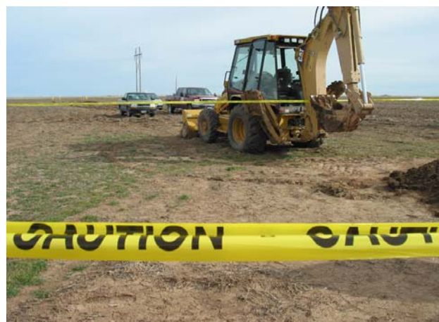
Excavation Event That Resulted in Cutting a Buried Electrical Line
