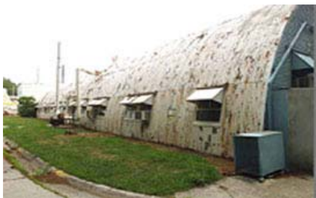
Deteriorated Quonset Hut
