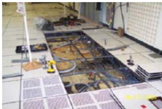
Exposed CO 2 Fire Suppression System
