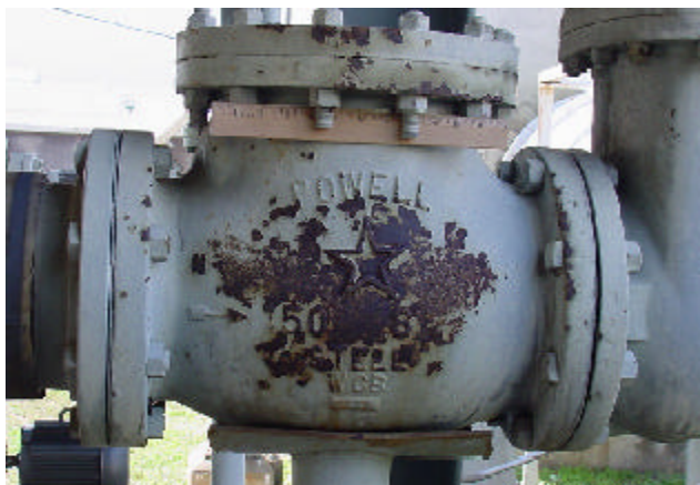
Damaged Backdraft Damper
