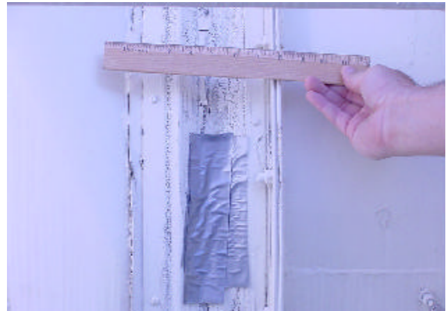
Flexible Joints Repaired With Duct Tape
