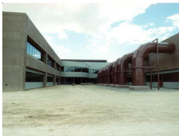
Ventilation Systems at MDL
