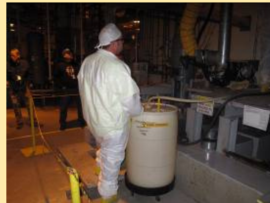
Draining of D2O from Shut Down Cooling - Nov.2, 2009
