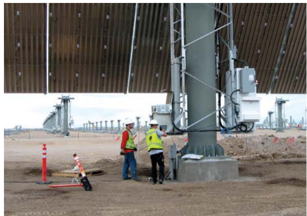
Workers testing the automatic stow-capability trackers for a concentrating solar photovoltaic module at the 30 MW Cogentrix solar power plant in Alamosa, Colorado.
