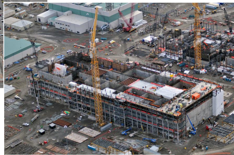
Pretreatment Facility (PT)
