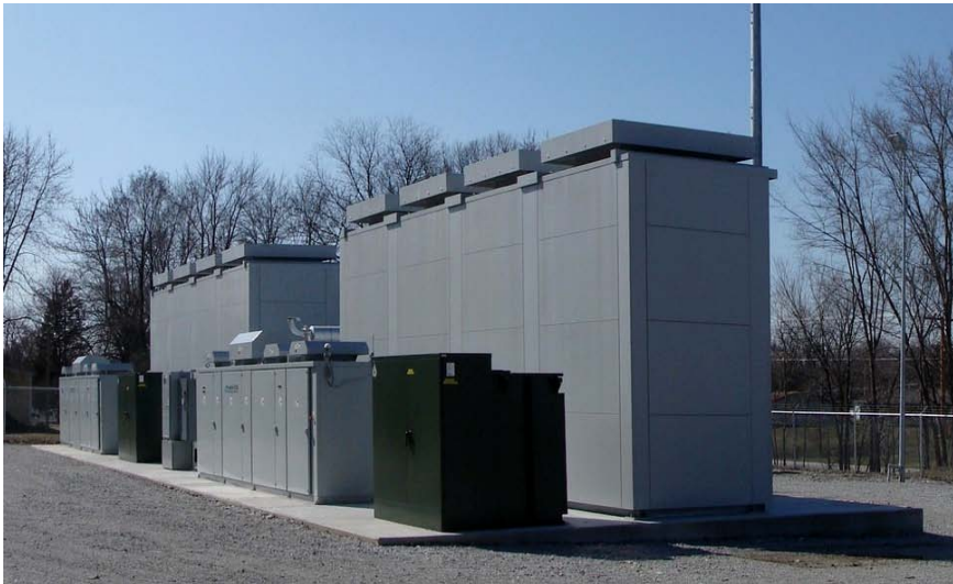
2MW, 14.4 MWh in Churubusco, IN
