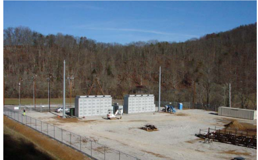
2MW, 14.4 MWh in Milton, WV
